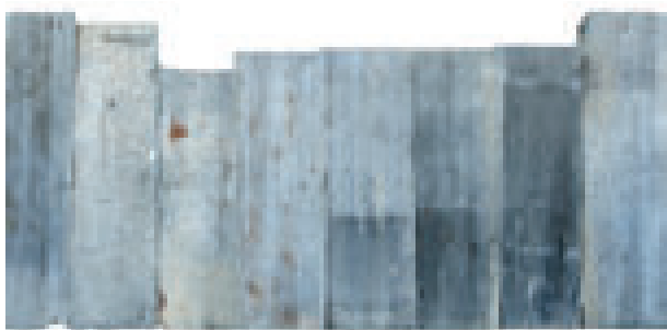
Fig 10.7 Damaged iron sheets
